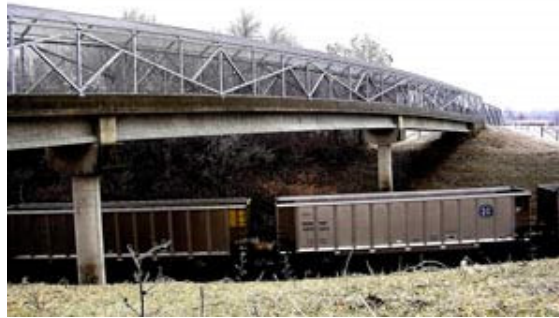
The Bridge serves as an important connector in the trail system by spanning this rail line
